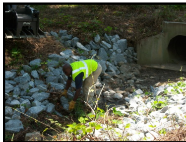
Cleared and properly stabilized, the culvert can safely serve its intended purpose.
